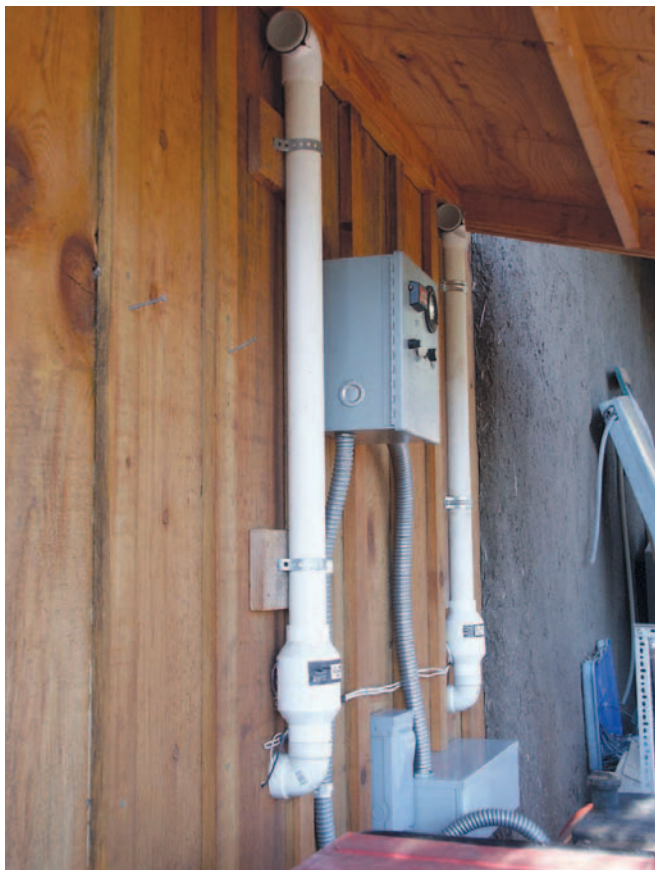
These two Zephyr battery vents safely pull hydrogen gas from the battery boxes (inside) to the outside.
